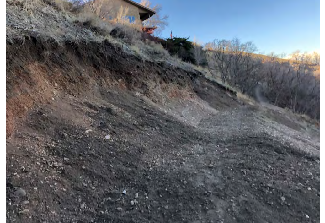
Inadequate slope analysis and design prior to construction resulted in excessive impacts.
