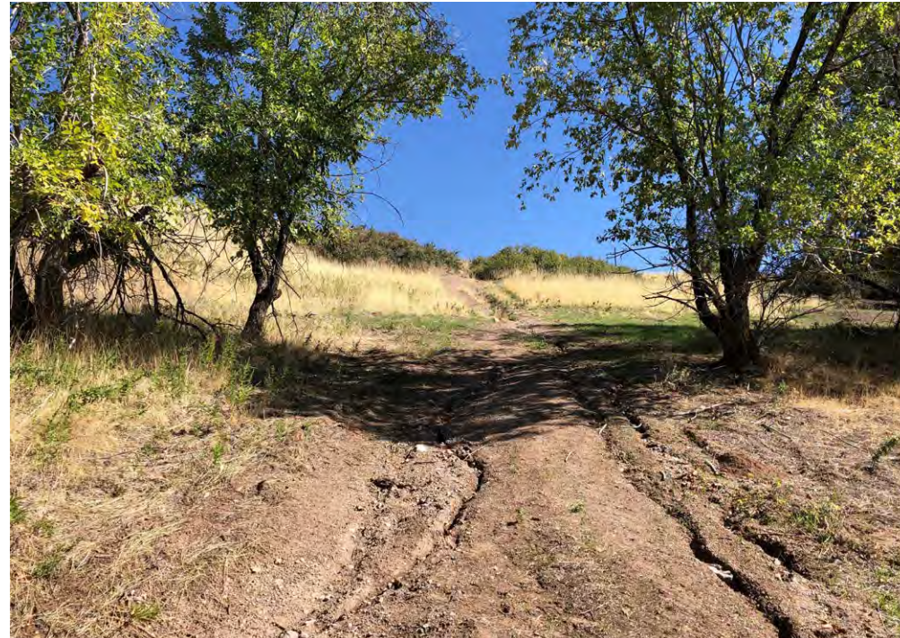
South Popperton erosion: South Popperton Walking Trail is textbook “fall line” trail that should be realigned to shed water and prevent erosion.
