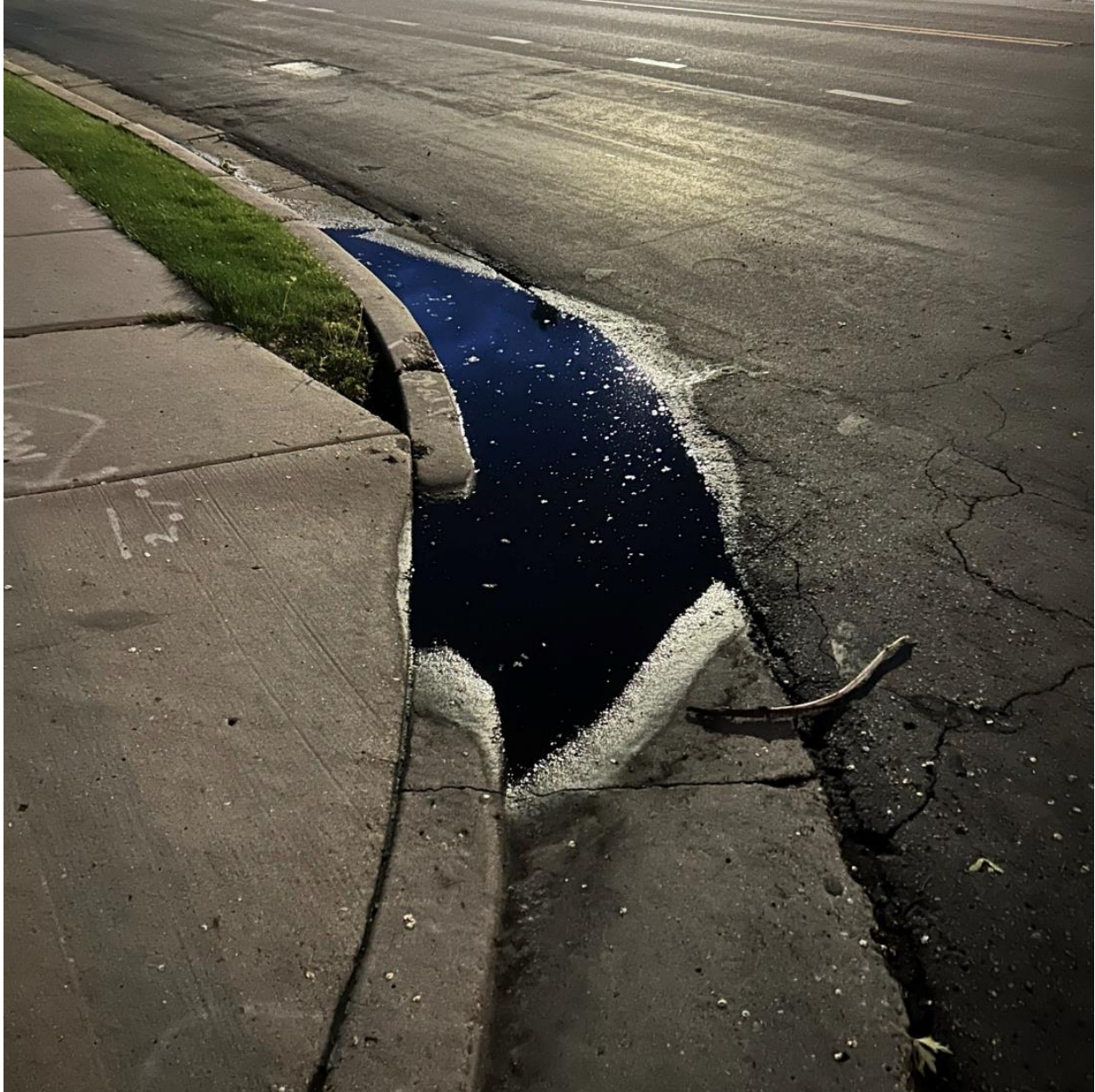
Photograph 10 – Water Pooling on Southwest Corner
