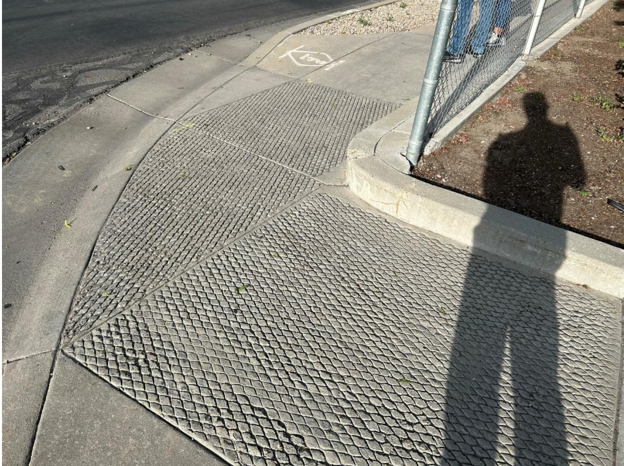
Photograph 7 – Pedestrian ramps do not meet current ADA standards
