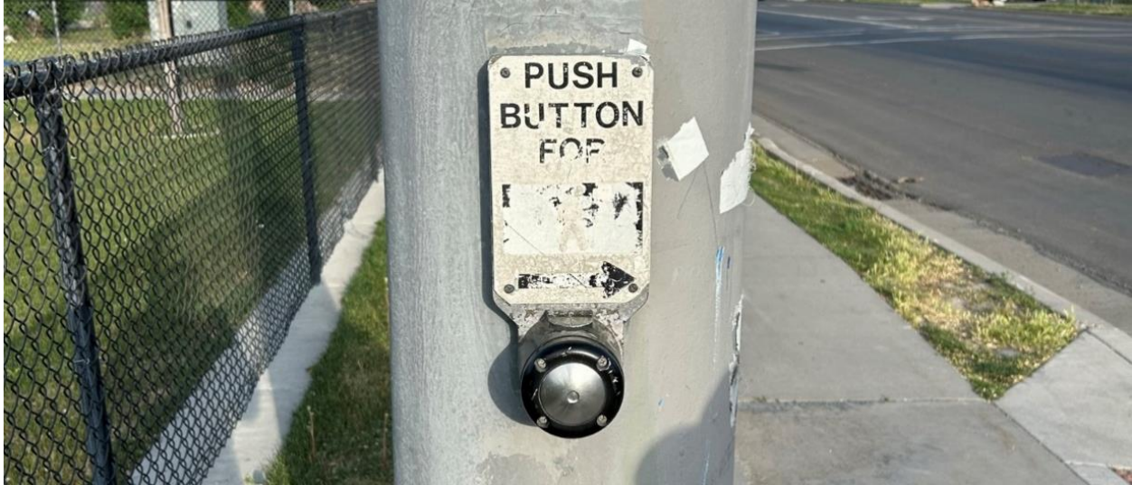
Photograph 2 – Example of Weathered Crosswalk Push Button Sign
