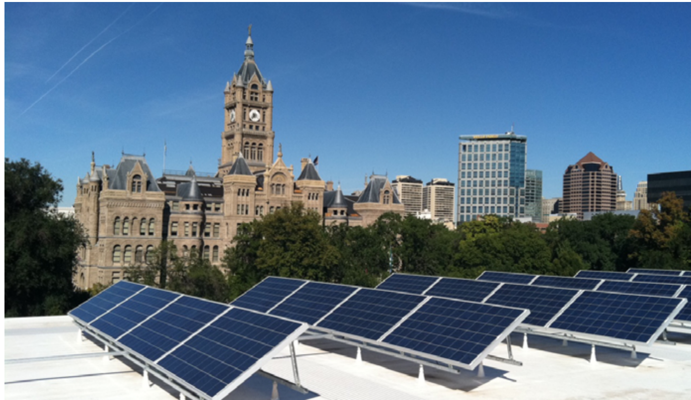
Solar panels installed on the roof of the Leonardo Museum in downtown Salt Lake City in 2016
