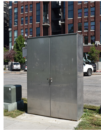
S12. Large electrical box
