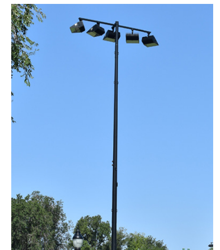
S9. Variation of field light pole
