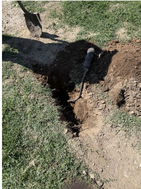
Improperly installed 8005 Rotor head
